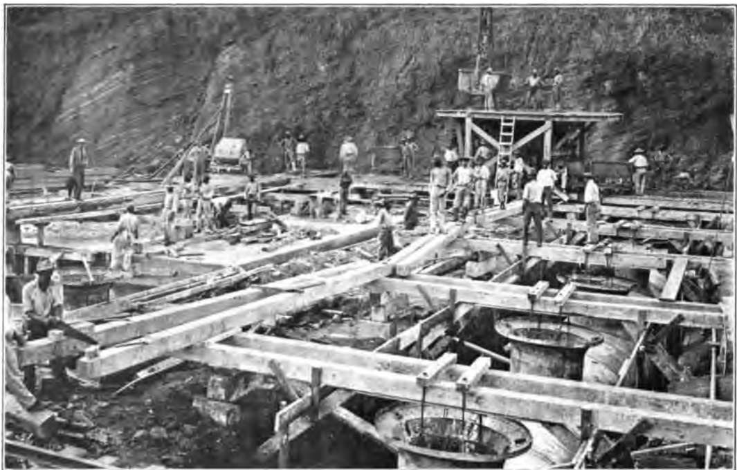
CROSS SECTION OF PEDRO MIGUEL LOCK, SHOWING LATERAL CULVERT FORMS IN PLACE, JAN. 5, 1910.
