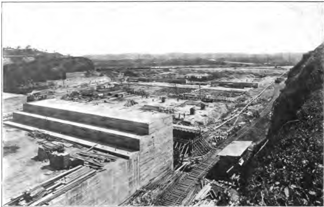
LIFT SILL AND FOREBAY, LOOKING SOUTH, FROM WEST WALL, GATUN LOCKS, FEB. 1, 1910.
